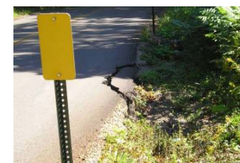
Richvale Road CR3, slip before repair
