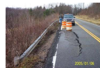
Shannon Road CR48, slip before repair
