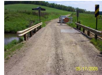
North Branch Rd before repair
