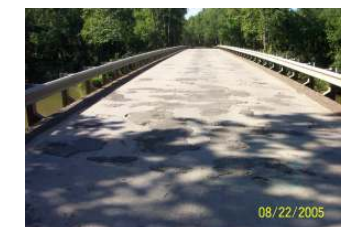
Pleasant Valley Road, bridge before repair
