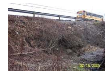
N River Road CR3, before embankment repair
